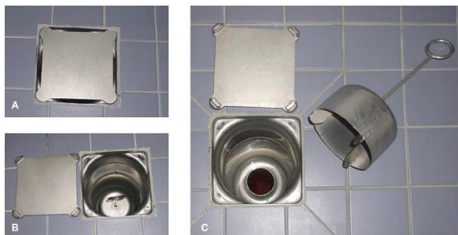
Figure 1. Shower drain design. The whole installation is covered by a heavy stainless steel lid (A), which is designed to discourage patients from opening and to prevent accidental removal. The drain (B) is designed to be wide, so it can be easily cleaned and disinfected. A bubble cap insert (C) prevents odors and splashing and can be removed for sterilization.
